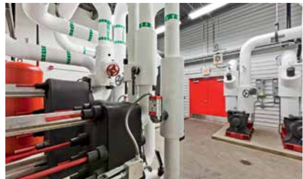
Plant room for turnkey acoustic testing facility
