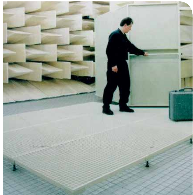
Example of Microdyne® fully anechoic chamber with cable floor plus additional platform for Deutsche Telekom
