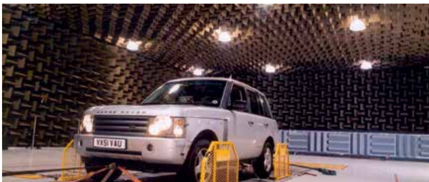
Refurbished anechoic pass-by chamber facility with foam and IAC Metadyne® wedges
